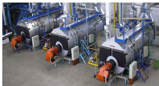
Fig.1. Central boiler house
