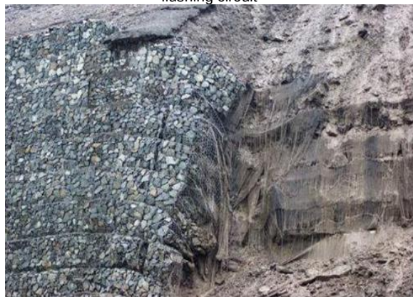
Figure 5. Breakdown of gabion retaining wall due to errors in design or installation of the structure
